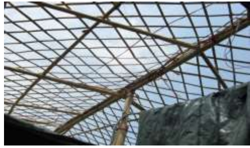
Storm damage hospital . Photo. S.Halbert May 2018
