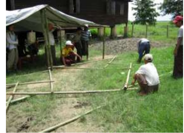
Laying out the two additional roof frames to mark the position of the support posts
