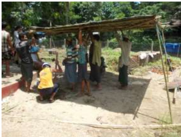
Holding the roof up while the support posts are dug is easy.
