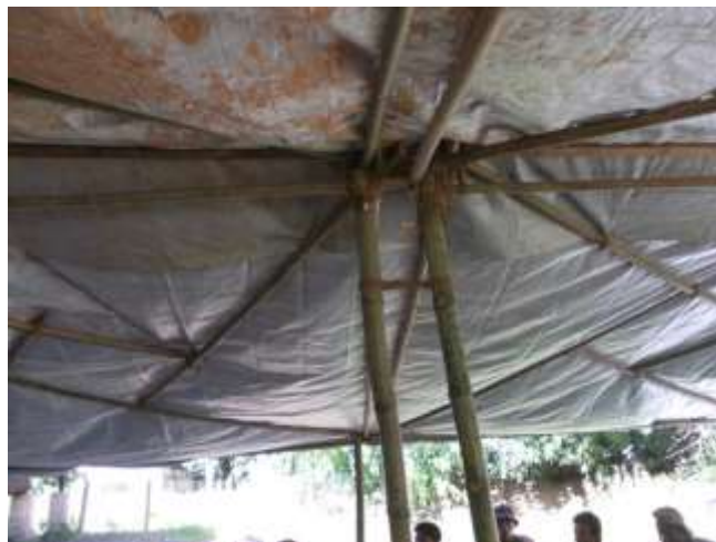
Double support poles work well. Note additional top ridge pole added to support tarpaulin
