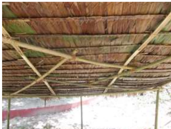
Loading is reasonably spread over the central frame. A third split bamboo pole lashed across the upper and lower intersecting frame points may be even better.
