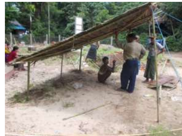
Shelter roof elevated. An additional central support has been added to the lower ridge pole.
