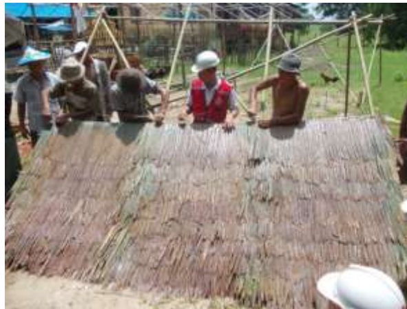
Frame support was remarkably flat with a good incline for water runoff
