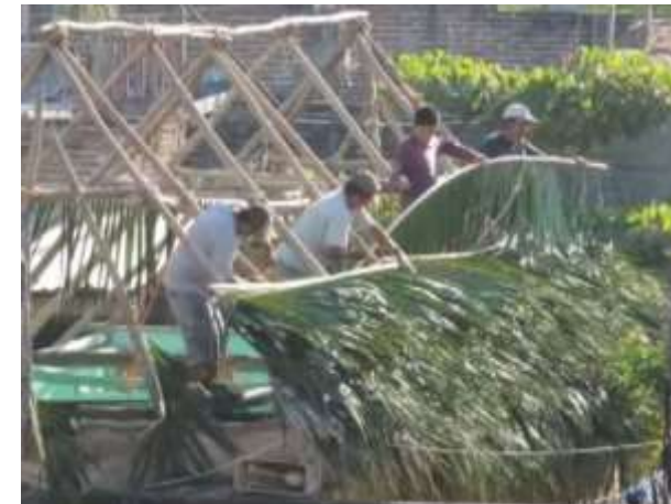
In an emergency split palm leaves, as used for thatching this permanent roof, would be layered from bottom to top.
